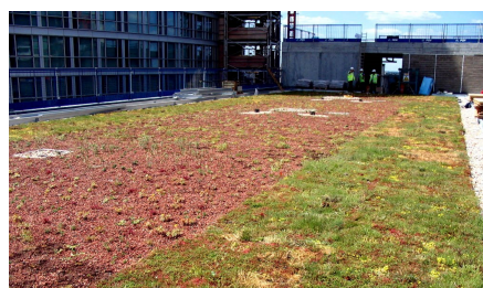
The vegetation mats laid along the roof edge provide instant ground coverage and from wind suction security.
