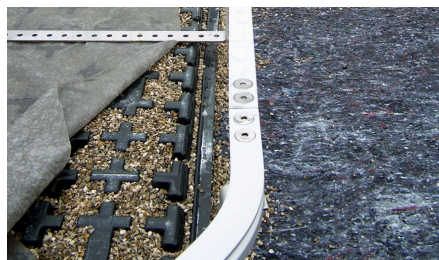
In addition, a rail system was attached to the SB 200 boards to protect against falls.
