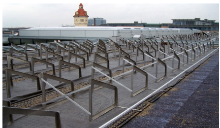
Each Solar Base Frame has been mounted on a 2 m 2 Solar Base Plate SB 200.
