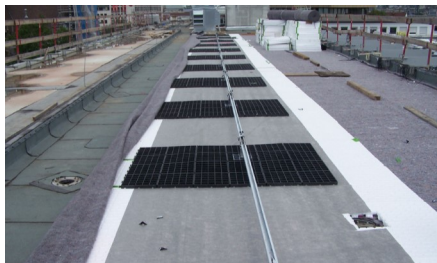
On the above green roof area was the fall protection system Fallnet® SR Rail installed.
