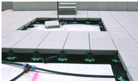
Under the elevated concrete slabs was enough space for the irrigation pipes.
