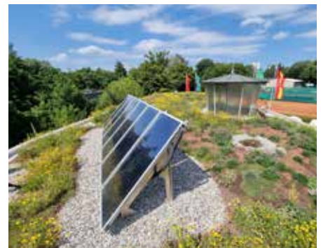
The green roof was combined with the existing solar energy unit – therefore producing synergy effects.
