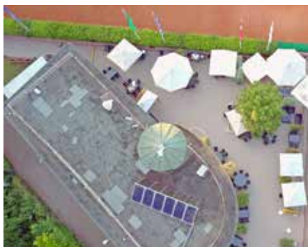
The KETV roof as a “naked” bituminous roof prior to the re-design as a green roof.
