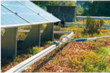
The fixing device in operation. The horizontal, gliding runner for personal protective equipment provides for maximum user friendliness.
