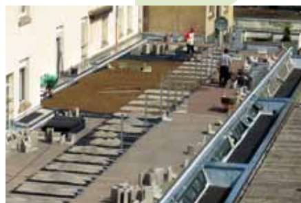
The elements are filled with grit for stabilisation purposes, which also acts as bedding material for the paving slabs which will be laid subsequently.
