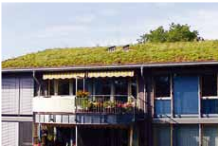
When dimensioning an eaves upstand or shear barrier, the decisive factor is not only the water-saturated weight of the green roof build up but also the estimated snow loads for the locality.
