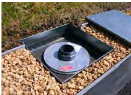
The flow controller is protected beneath the inspection chamber and regulates the slow discharge of water. At the same time, it acts as an overflow.
