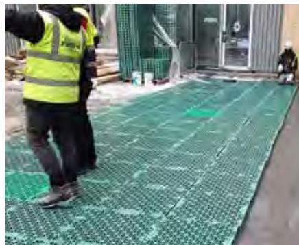
The heavy duty RSX spacers were laid on all podiums allowing them to be used as roof gardens with hard and soft landscaping.
